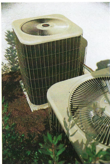
Figure 7 This air-conditioning unit keeps a building cool by moving thermal energy from inside the building to the outside.
